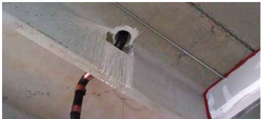
Blockouts were cast into some of the double tees to allow penetrations that plumbers could connect to an elbow, allowing plumbing to remain set in the design. Photo: FDG Inc.
