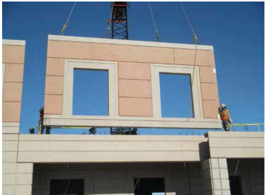
Panels feature several colors, reveals, and a variety of cutouts. Combining colors and textures into one panel reduced the piece count and sped up the erection process. Photo: FDG Inc.
